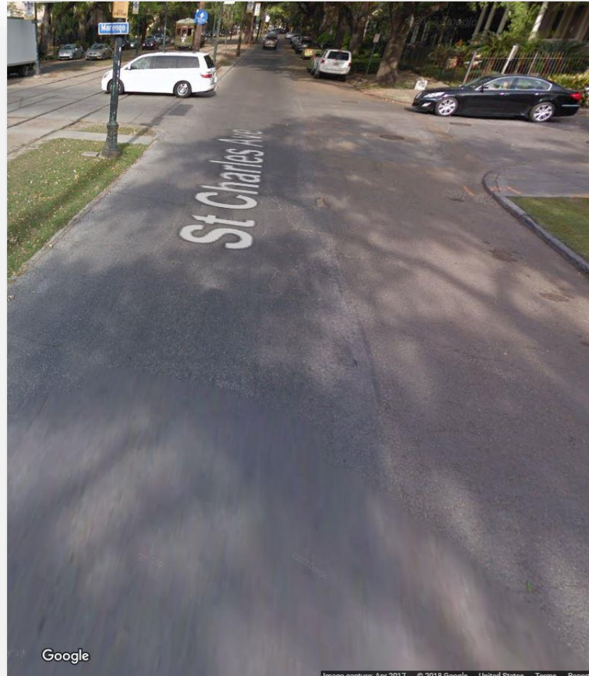
Existing condition at St. Charles Ave. and Marengo St. Pavement Condition Index is Poor.
